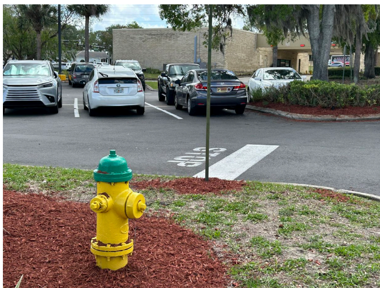
Figure 3 – Existing Fire Hydrant Near Proposed Parcel
