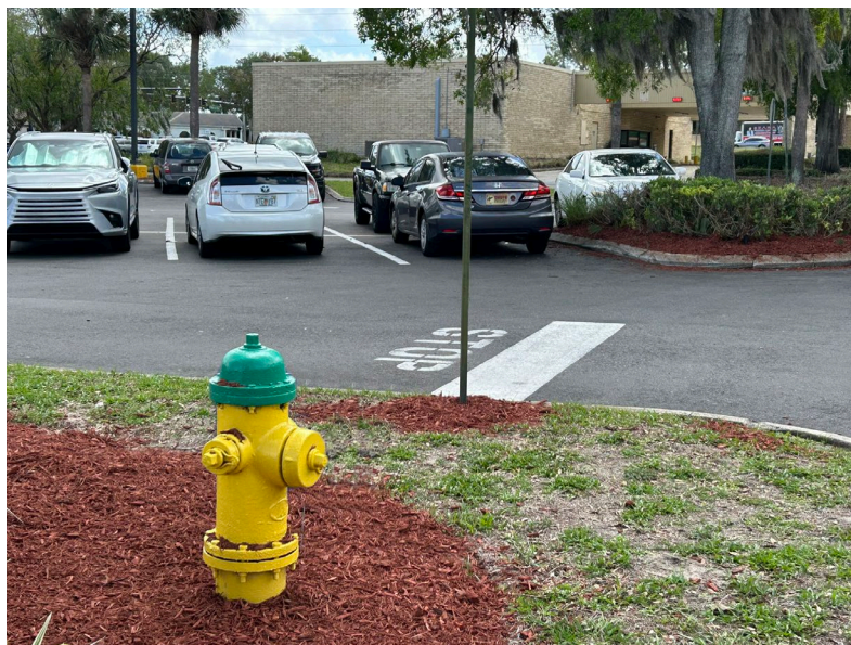
Figure 3 – Existing Fire Hydrant Near Proposed Parcel
